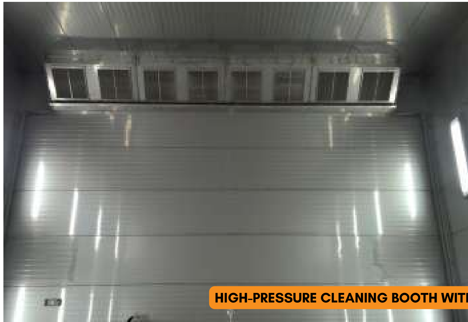
High-pressure cleaning booth with vapour extraction system
