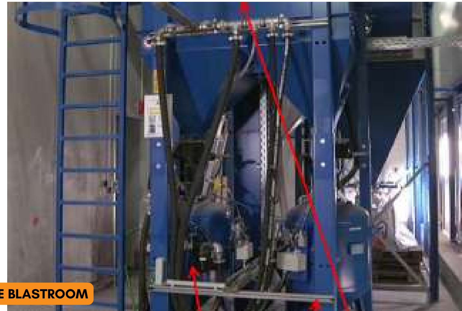
Two pressure blast pots / Media silo
