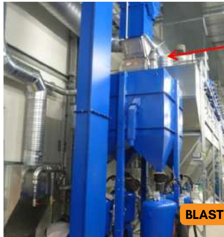
Machine room with filter unit
