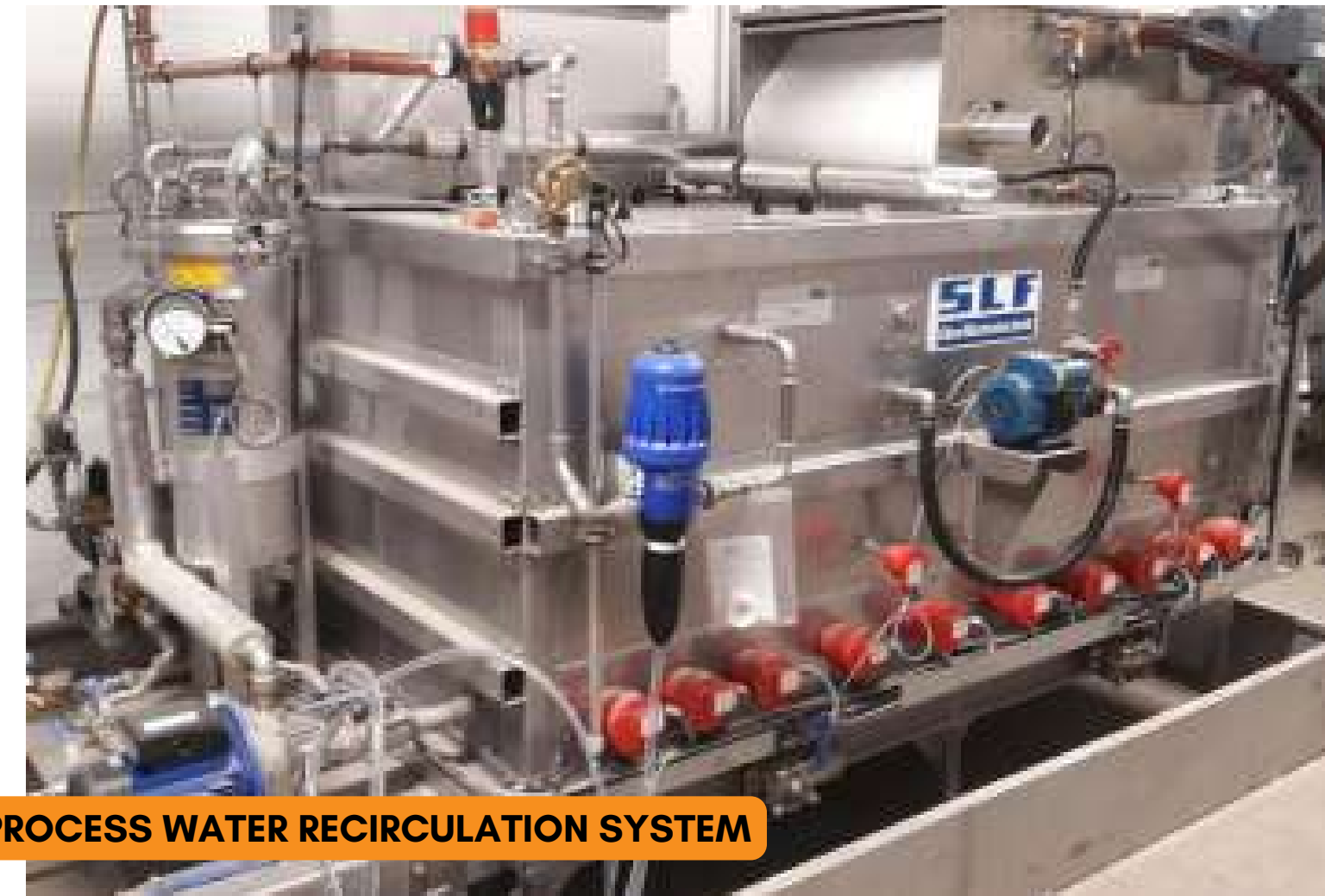
Process water recirculation system
