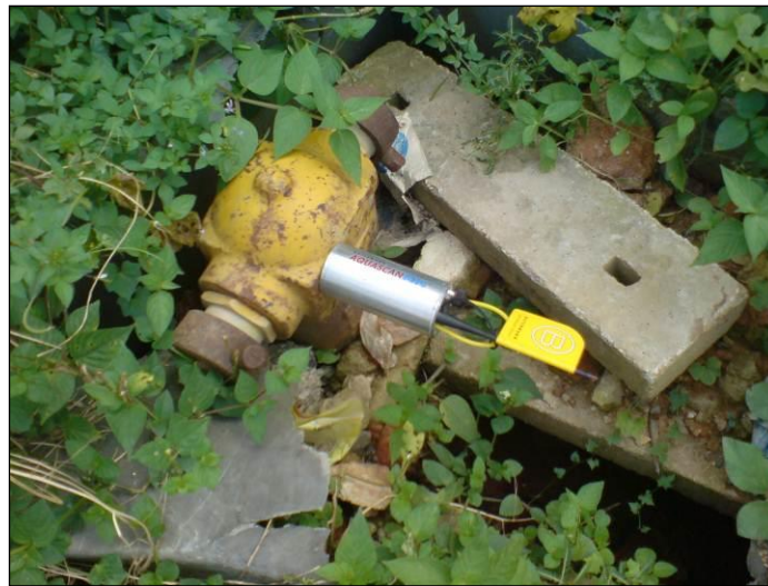
Fig. 48 the 'A' Sensor attached to a hydrant spindle
