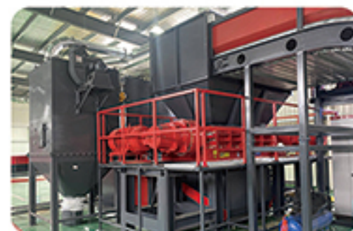
Material: Electric Waste Solutions: Shredder Area: SHANGHAI
