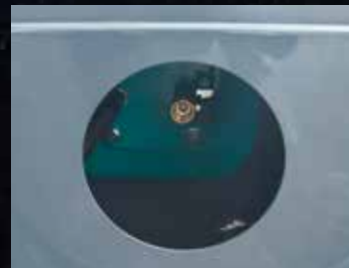
Remote fuel tank drain valve
