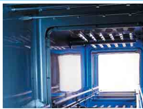
Washing chamber without internal pipes.
