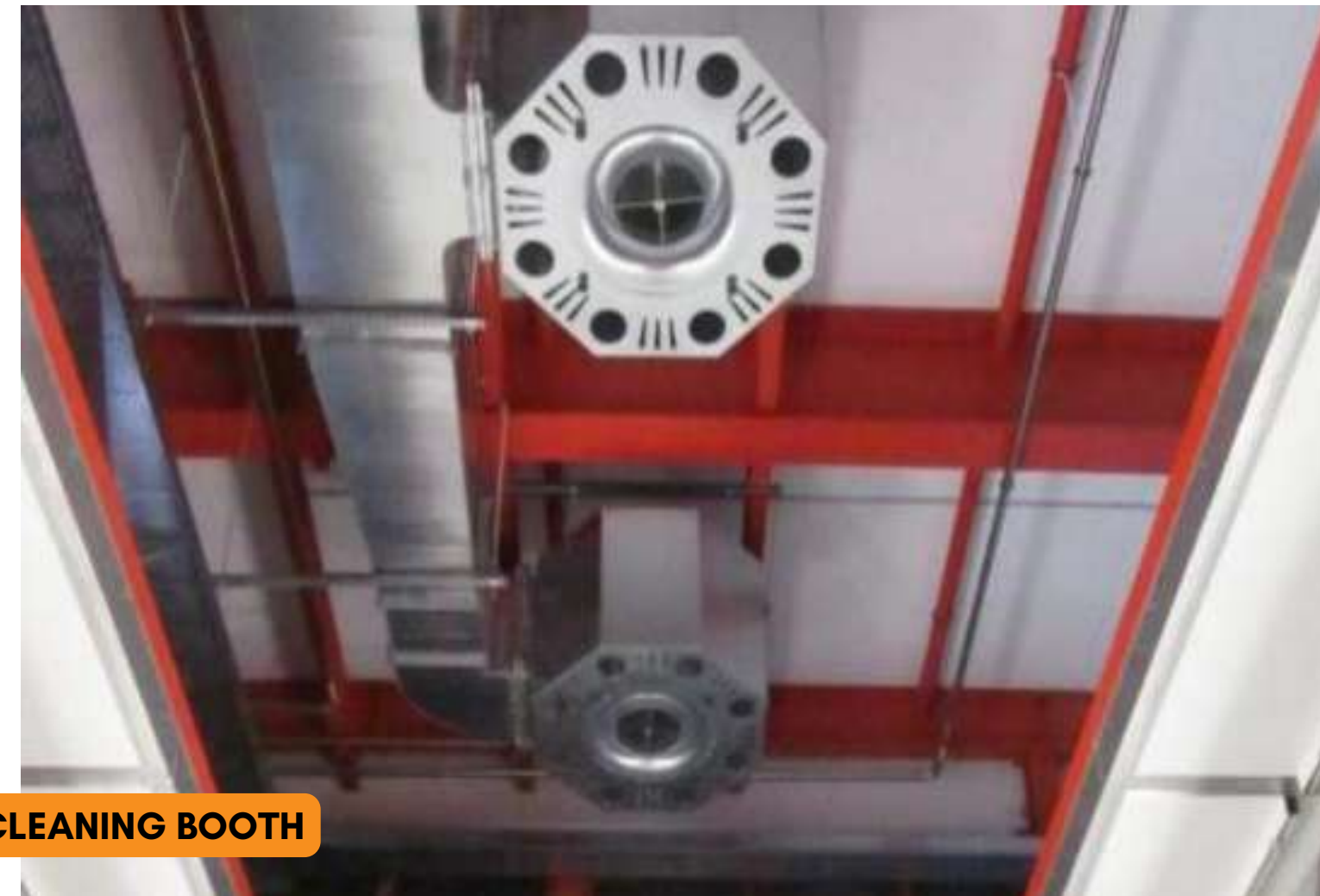
Permanently open crane slot
