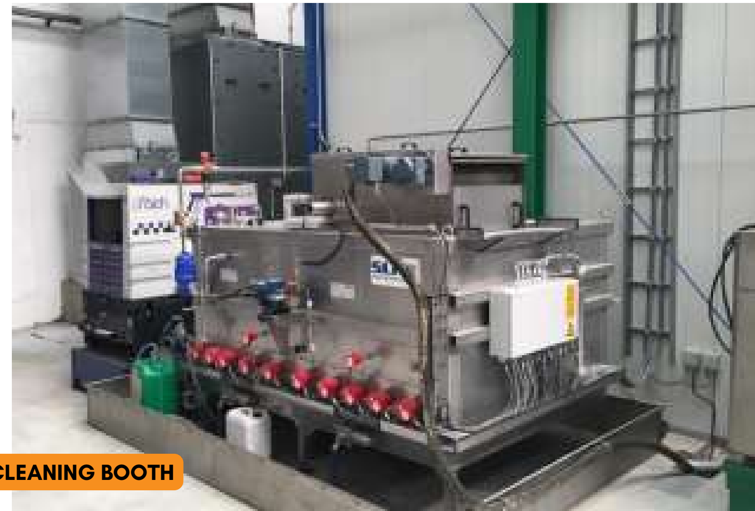
Process water treatment system
