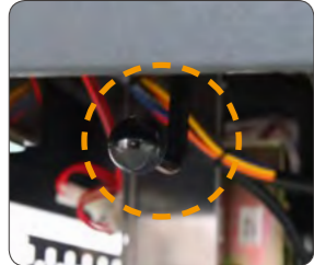
Manual switching lever on the control panel Enabling driving for narrow space or when the battery is discharged.
