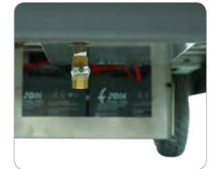
Condensate drain valve
