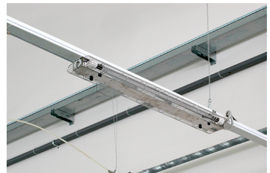
Application in an industrial environment
