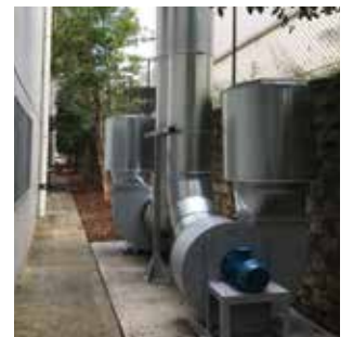
22.5kW and a 15kW Fan
