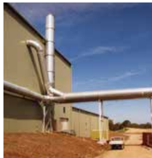
Vertical Discharge Stacks
