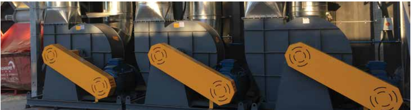
3 x 75kW High Efficiency Centrifugal Fan installed on a large dust collection project in Sydney
