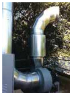
30kW High Efficiency Centrifugal Fan
