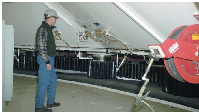
The raised roller path of P&H draglines provides ample space for inspection and component changeouts.
