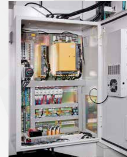
High quality electrical components and circuits are fully protected. Neat wiring arrangement is easy for maintenance.
