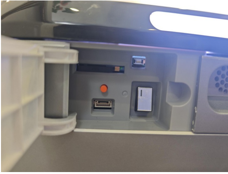
Main switch, pairing and service access area
