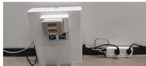
Charging station placed against the wall
