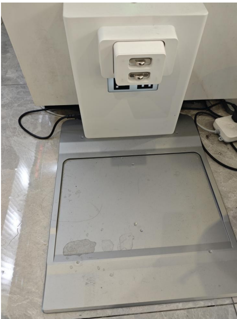
Charging station fixed to base plate
