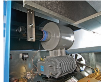
View with rear panels removed.
