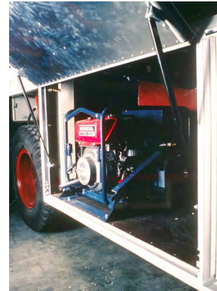
Generator and compressor in heated compartment
