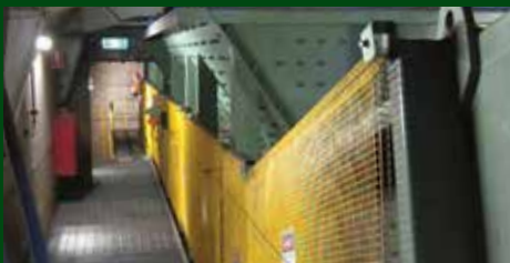
LPF™ beneath rail line at a port installation handling iron ore at 3000tph.
