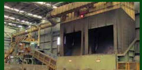
1500tph concentrate feeder at Bunbury Port.
