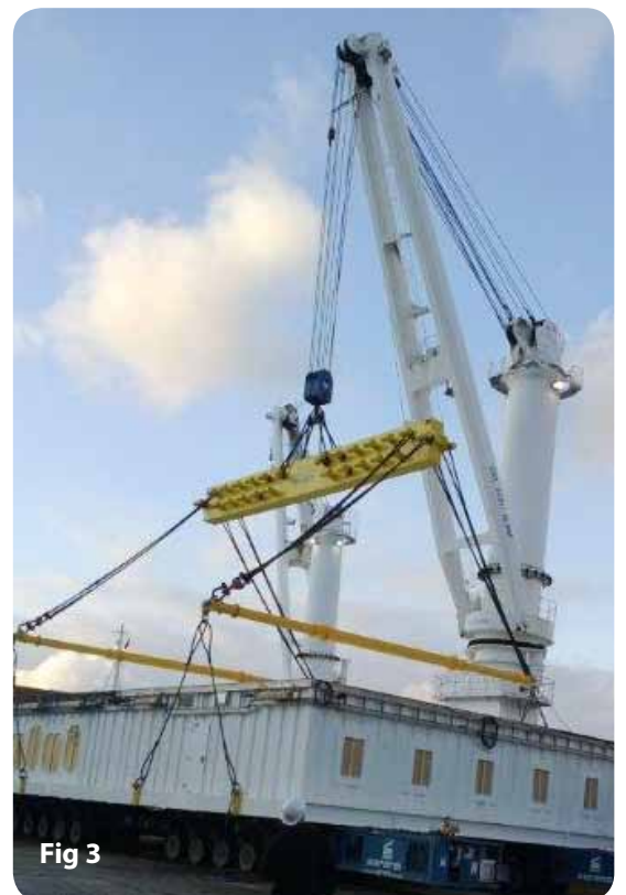
Fig 3: Skid being lifted by 2 x Spreader Beams and a single Lifting Beam
