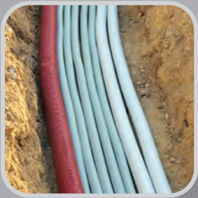
Electric Power Lines
