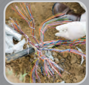
Telecommunication Lines and Fiber Optics
