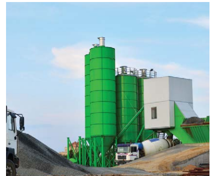
Cement Batching Plant
