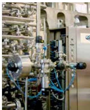
Recycling valve group
