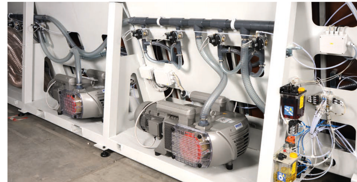
Dry vacuum pumps (Made in Germany)
